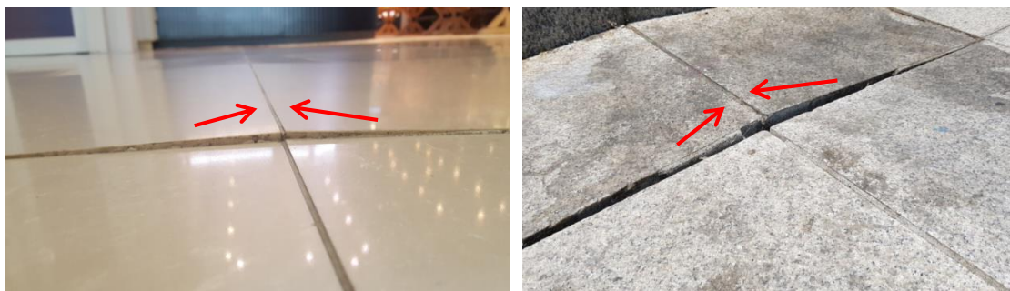
< Expansion problem case: Left: E-stone, Right: Natural stone >
